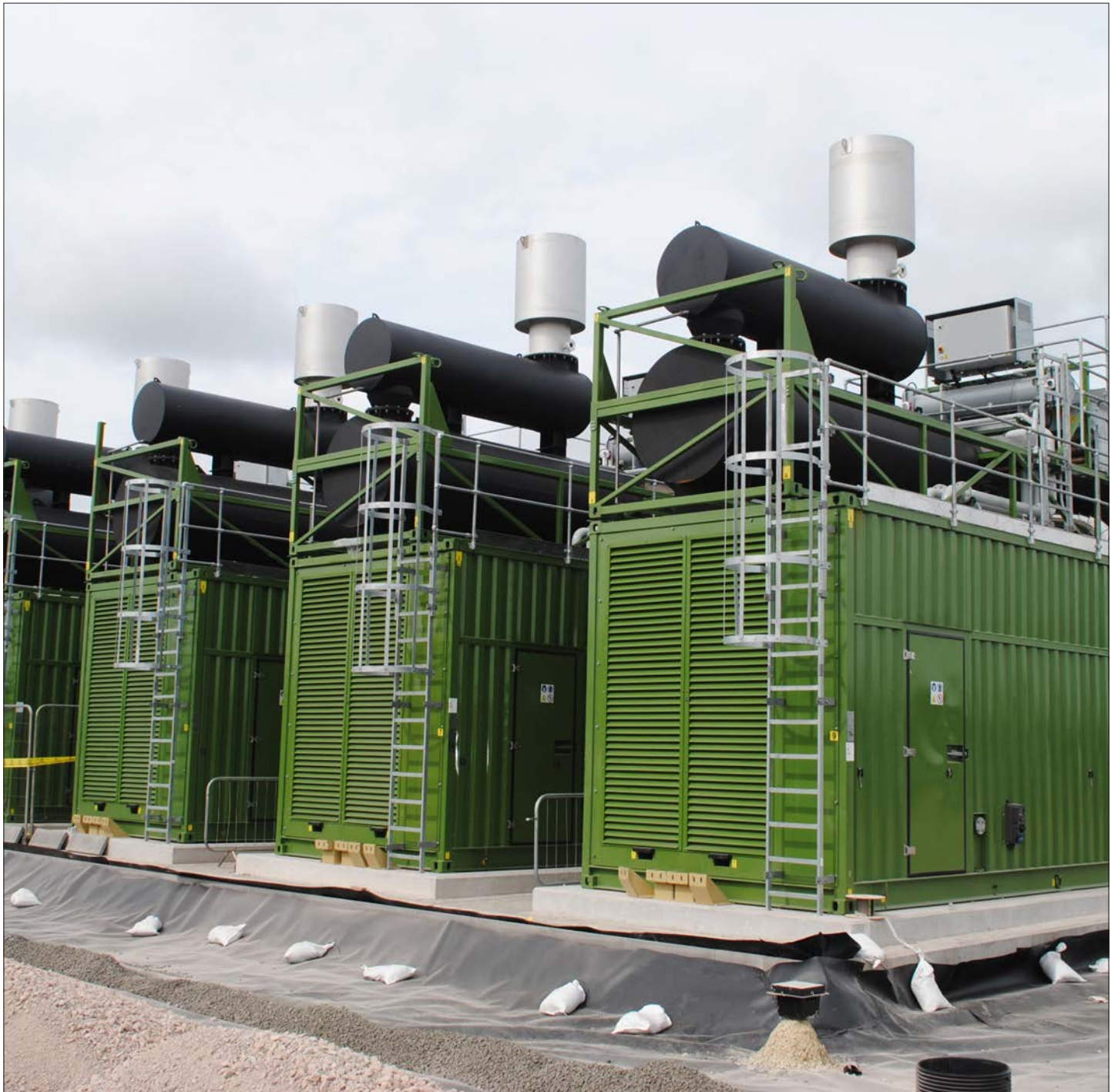
Above: One of UK Power Reserve's battery storage sites
