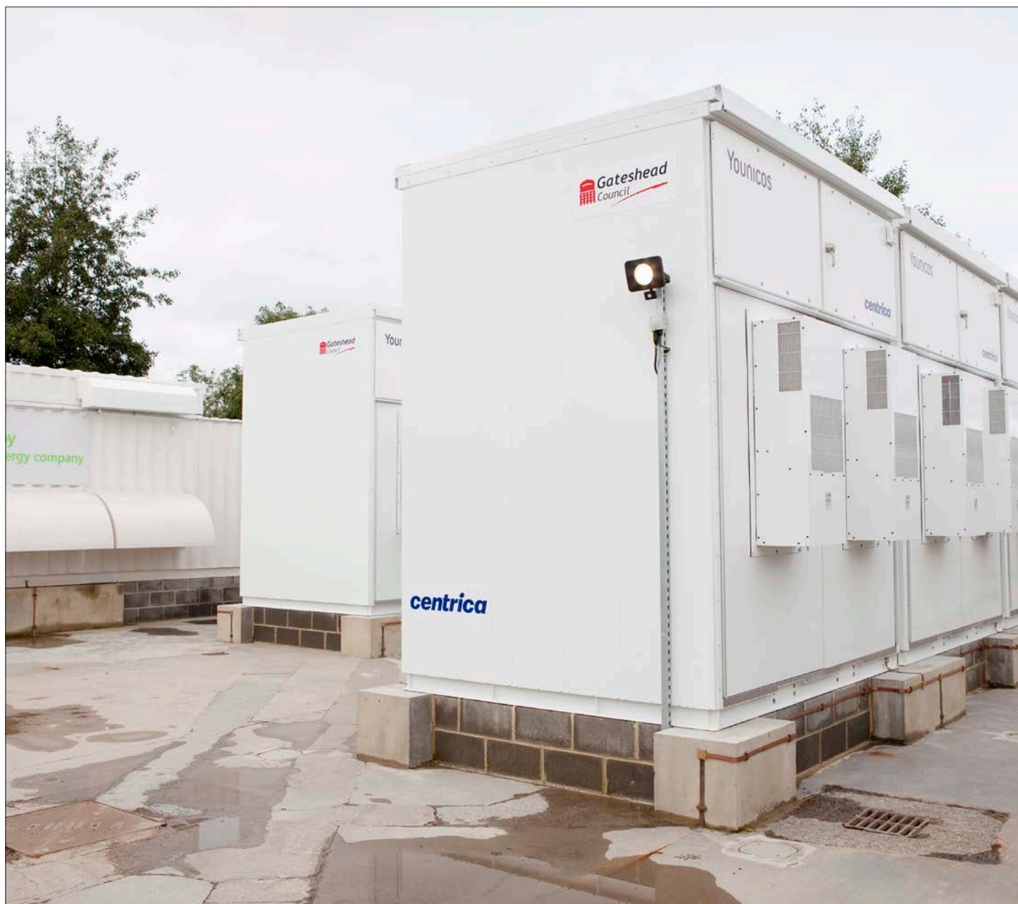
Above: Battery storage installed as part of Centrica's relationship with Gateshead Council
